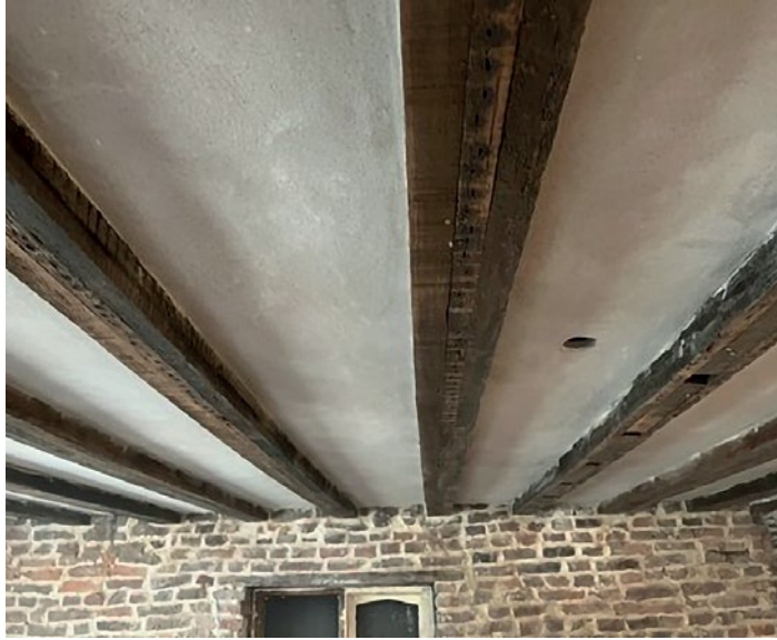
THE painstaking work to restore and recreate the historic Raven Inn at Glazebury, saved from demolition by local campaigners, can now be revealed.
