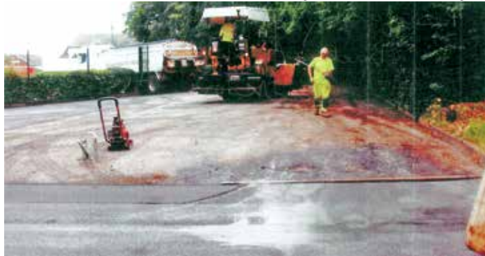
Resurfacing the activity area at the back of the Scout Centre on Jackson Avenue.
