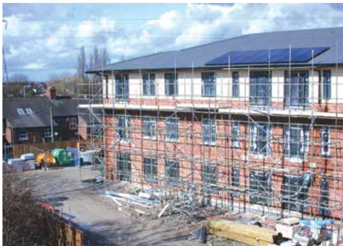
A £9.5 million community care village being built in Warrington has celebrated a key milestone with a topping out ceremony to mark completion of the roof and main building work at Belong Warrington.
