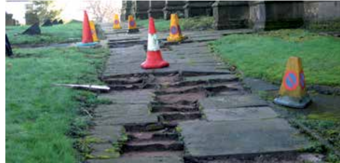
The damaged path where the flagstones were stolen.
