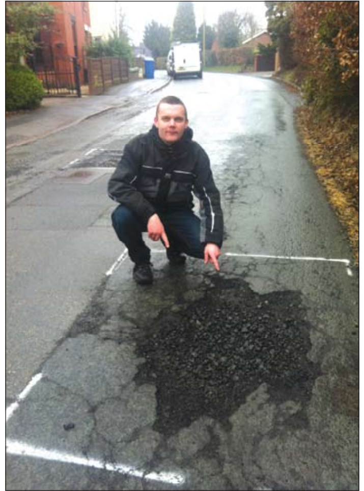
Cllr Smith highlights the damaged road surface at Fowley Common.
